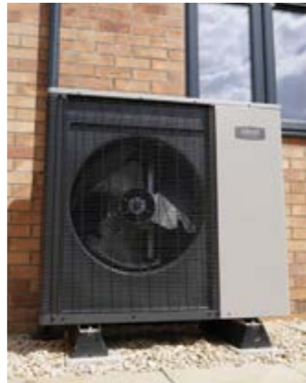
Air source heat pump in every home.
